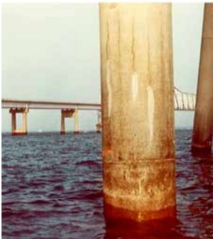
▲ Example of pile "scour"
