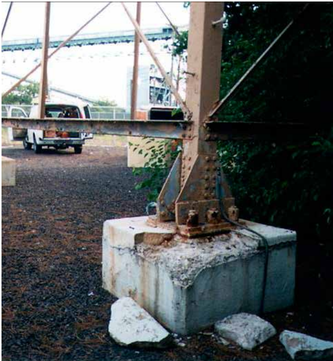
Severe damage to concrete foundation
