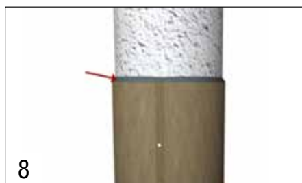
8 Install FX-763 Low-Modulus Trowel Grade Epoxy at the head of the jacket and finish to a 45° tapered bevel, creating a water- and chemical-resistant barrier to the repair system.
