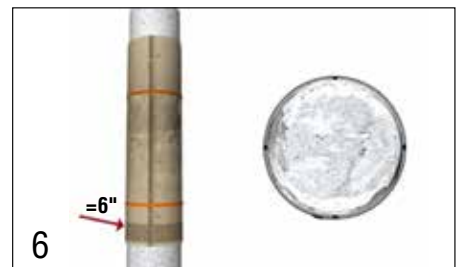
6 Install 6" (152 mm) of properly mixed FX-70®-6MP Multi-Purpose Marine Epoxy Grout to create bottom seal; allow grout to cure overnight.
