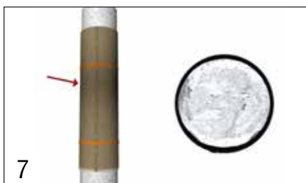
7 For piles with ≤ 25% section loss, fill remaining void in jacket with FX-70®-6MP. For piles with > 25% section loss fill void with FX-225 Non-Metallic Underwater Grout, leaving 4" (102 mm) open at head of jacket. Allow repairgrout to cure overnight. For FX-225 repairs, fill remaining 4" (102 mm) void with FX-70®-6MP, and allow grout to cure overnight.
